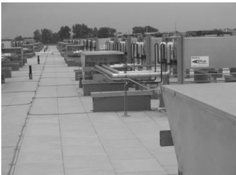
Here is an array of bonding jumpers. NFPA 780, the Lightning Protection standard, requires bonding metallic objects on the roof to prevent flashovers. But if you limit this bonding to objects on the roof, you endanger electronics in the entire facility. Consult your electrical contractor before finalizing a project plan.
